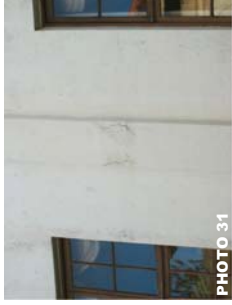
PHOTO 30 NORTH WALL, 2ND LEVEL FLASHING SPALL AT A-6
