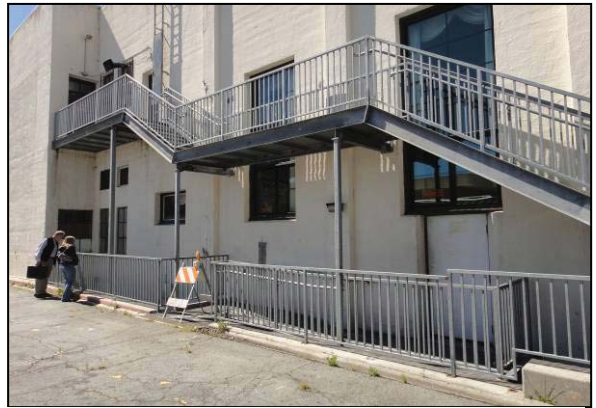
Fire escape stairs
