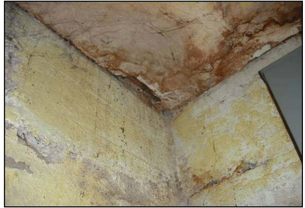
Interior spalling & stain ceiling
