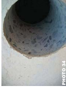
PHOTO 33 SOUTH WALL, 2ND LEVEL CORES AT D-6.3
